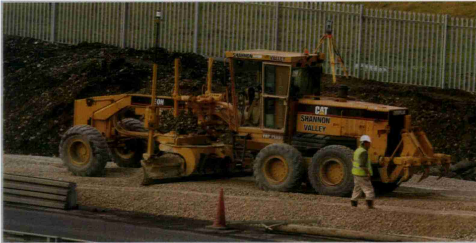
Shannon Valley Hire has supplied much of the equipment for the widening of the M50 including graders, such as this Caterpillar 160H, and more than 60 excavators.
